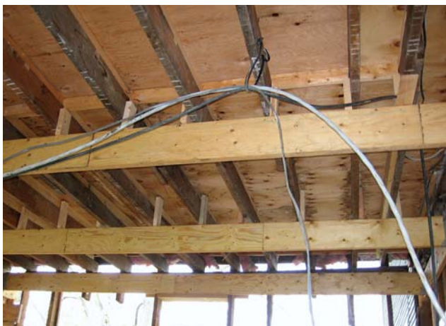
Figure 1. A new 14-inch LVL beam, inserted below the existing second-story joists, spans the 24-foot-wide kitchen ell (top). Several smaller LVLs run between the beam and a ledger attached with LedgerLok screws to the main house wall (center). Short blocks between the LVLs and the original floor joists above help to stiffen the floor system (bottom).
