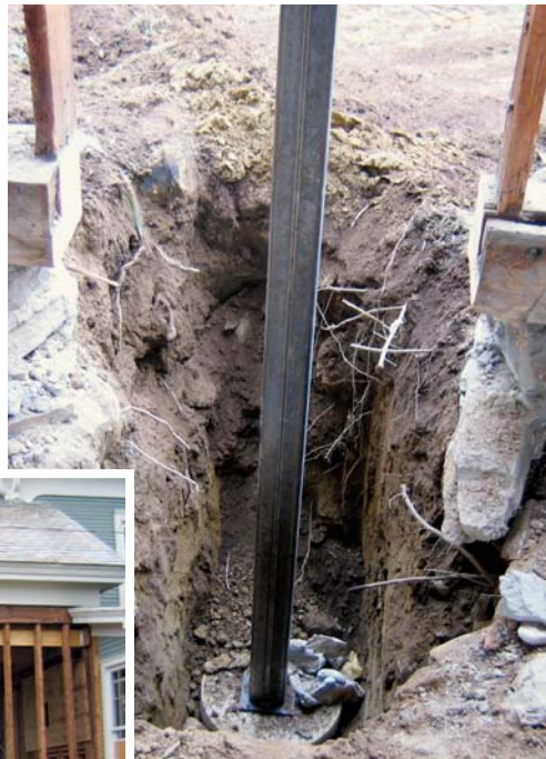
Figure 3. Working in increments around the perimeter, the crew removed as few studs as needed to excavate and install the steel posts (left). At the top, the studs were cut flush with the LVL ledgers and solid blocks inserted to provide good bearing for the 6-inch-square post caps (far left and bottom).
