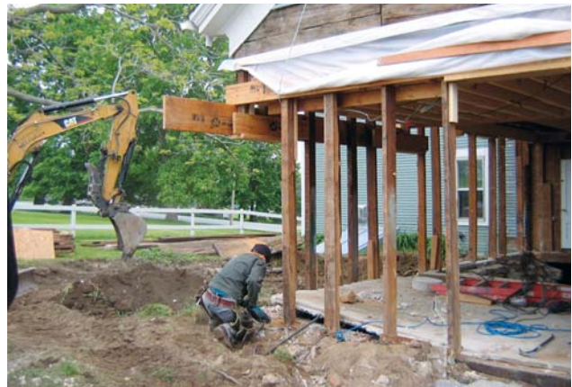
Figure 2. At the end of the ell and across the gable, wide LVLs are fastened to the outside face of the studs to pick up roof and floor loads when the walls are removed.
